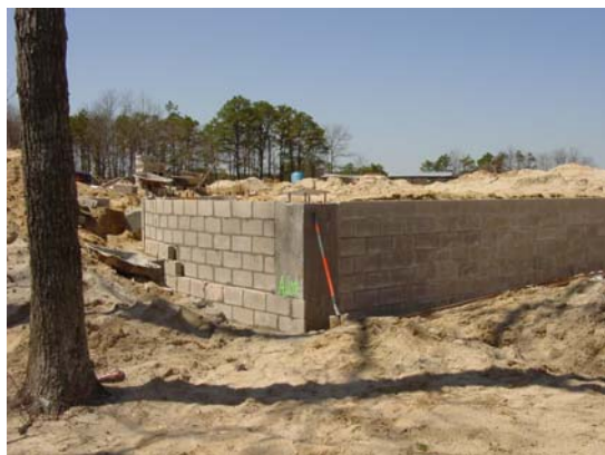
A retaining wall is under construction for ACCC's Cape May County Campus.
