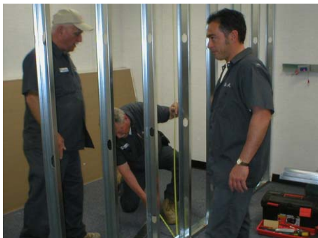
Facilities Management is hard at work renovating the Mays Landing East location (Building T). Installing walls for a computer lab are, from left, Dominick DiPietro, supervisor; Bud Ireland and Domenic "Ace" Acilio.
