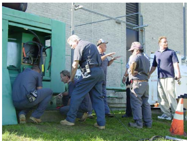
Facilities management staff troubleshooting the back-up generator
