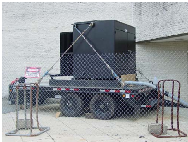
This emergency transformer outside K building will remain there while the regular K building transformer is being rebuilt.
