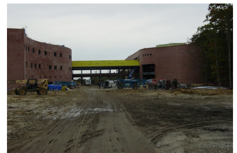
Exterior walls take shape as crews move ahead on Cape May County campus.
